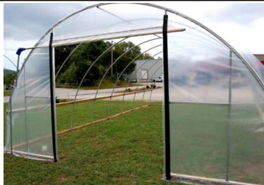
Finished Roll Up Door
